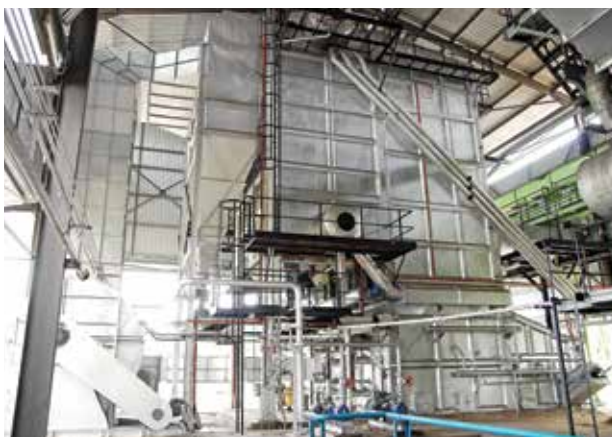
35TPH Palm Oil Mill Boiler
