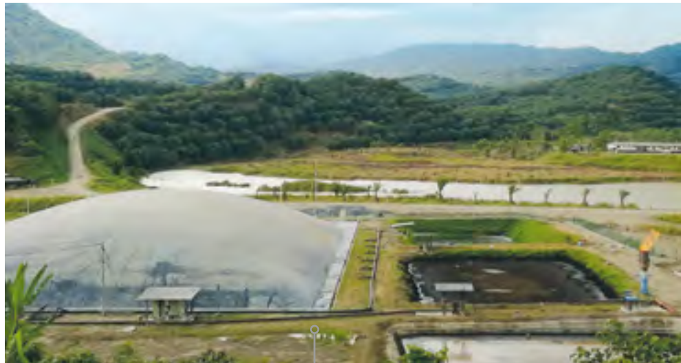
TEK MCLplus - Modified Covered Lagoon for Efficient Biogas Management
