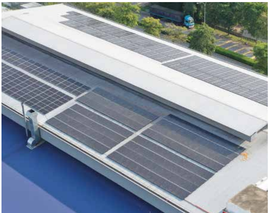
Tera - Commercial and Industry Solar PV system.
