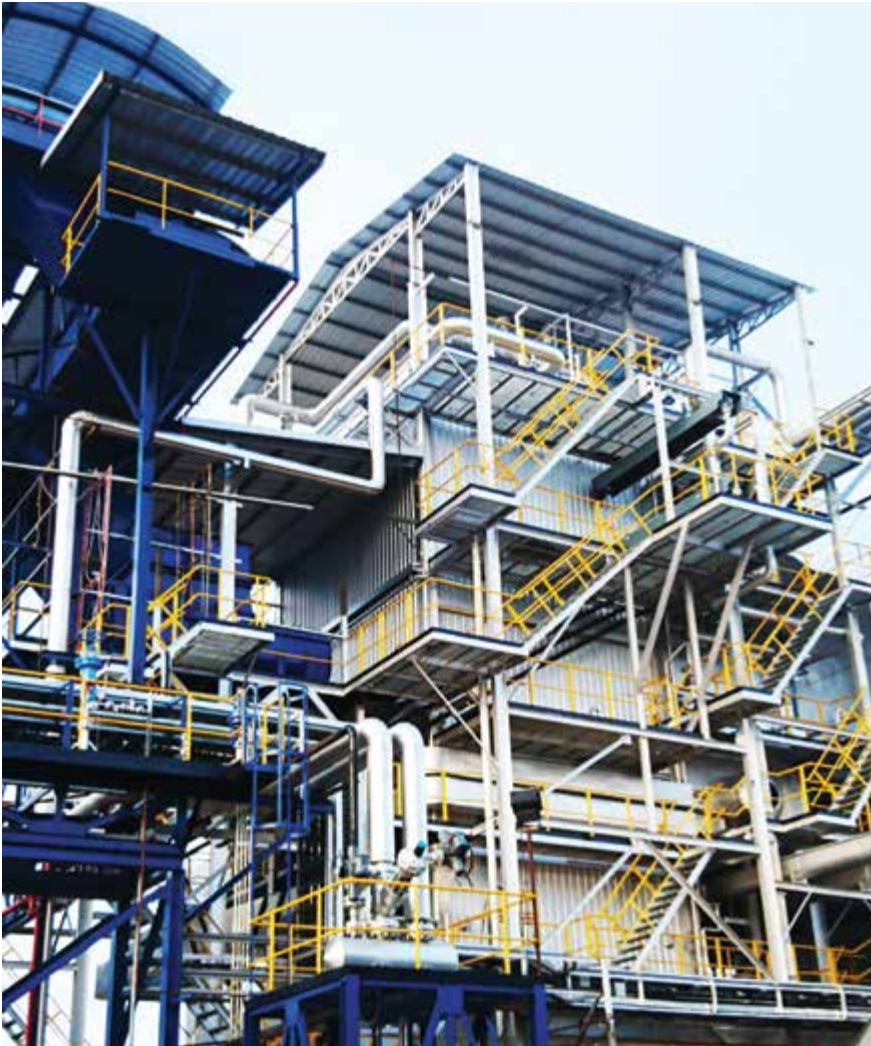
Outdoor type power plant boiler with ESP
